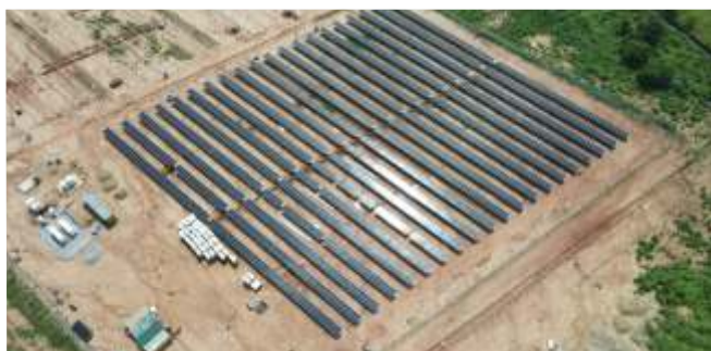
Solar installation at the 2,500 KWp Ibadan solar power farm.
